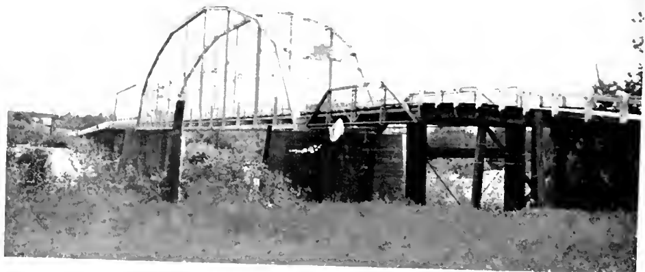
A "must" bridge which is weak and structurally unsound
